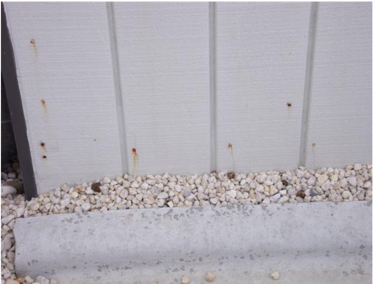
FIGURE ONE: Corroded Fasteners in Preservative Treated Plywood Cladding
