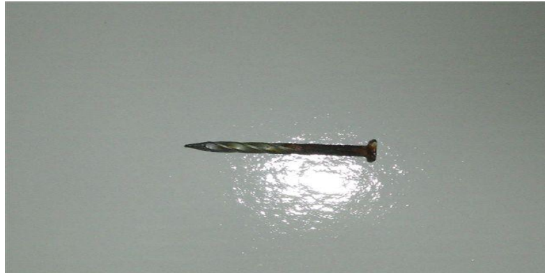
FIGURE TWO: Corroded Poorly Galvanised Nail – Extracted from Plywood Cladding – Unsuitable for Use in Exposed Treated Plywood
